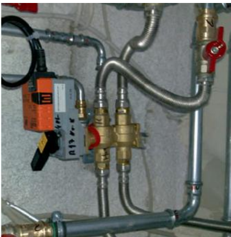
A 6-way characterised control valve (CCV) after installation (behind a suspended ceiling in the corridor area)
