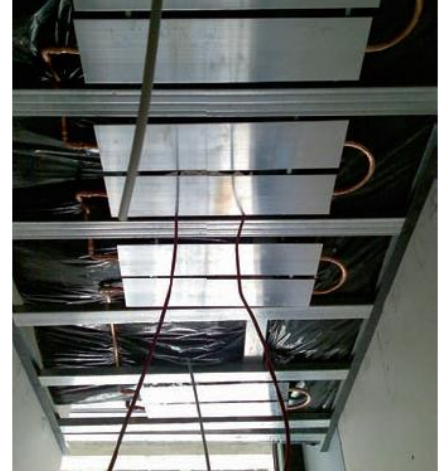
The heated/chilled ceiling elements are located behind a perforated suspended drywall ceiling
