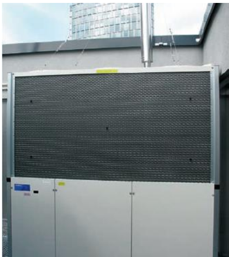
Three natural gas-operated reversible heating pump/cooling machines are used for the generation of heating and cooling performance at the Westpol building (installation on the roof)
