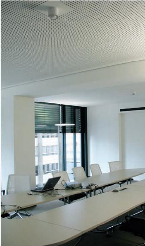
In the Westpol building, all of the office and conference rooms are equipped with combined heated/chilled ceilings and are supplied with conditioned supply air
